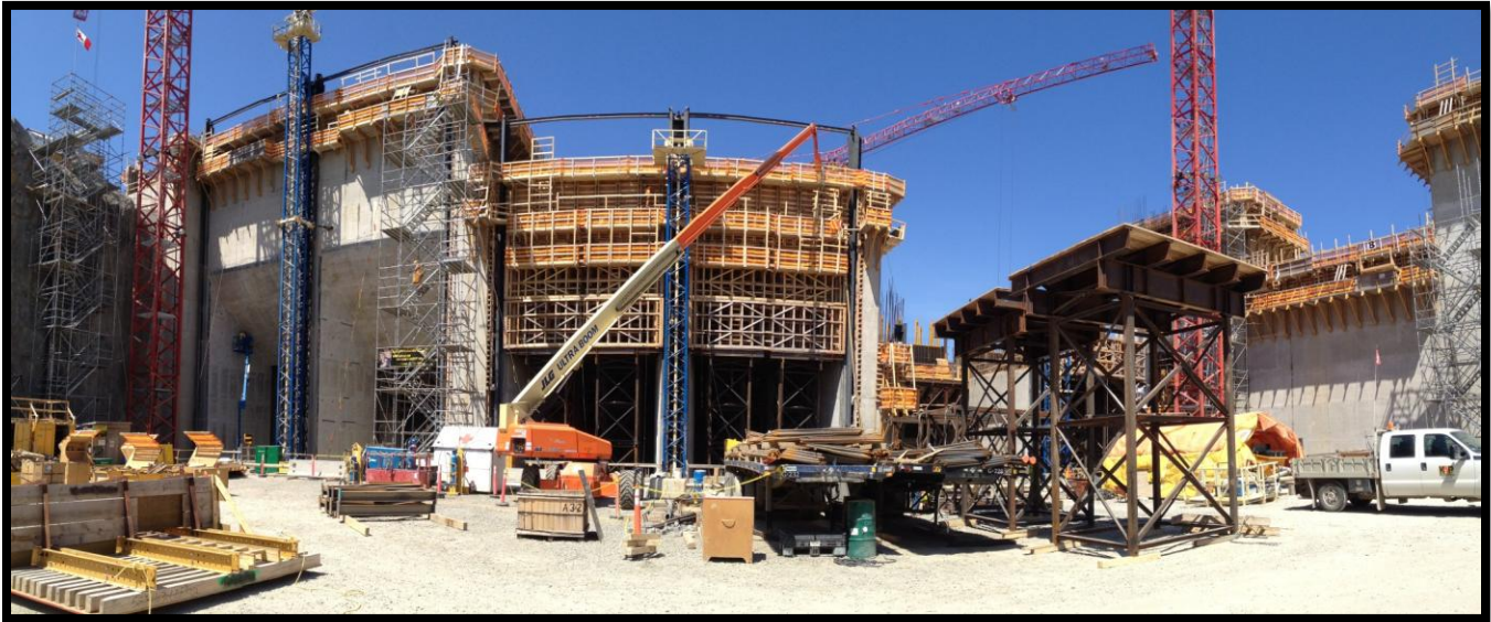
Figure 3: Smoky Falls Intake Overview
